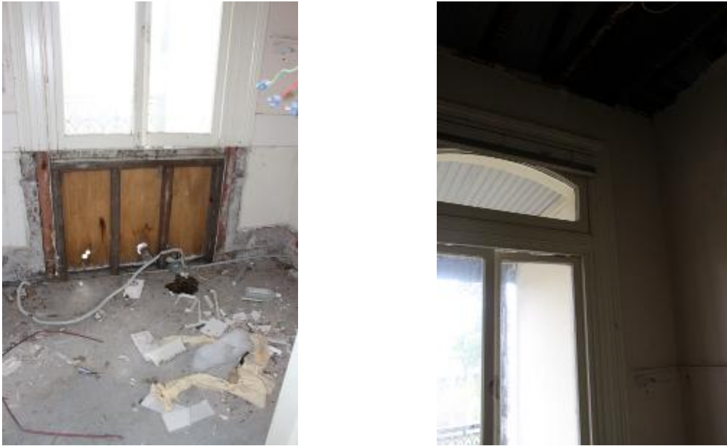
Figure 33: Part of Space F1 – recent enclosure & door converted to window
